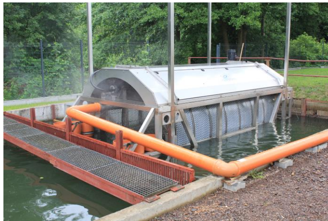
Figure 5. Drumfilter before installation AquaSyste Typ 200, such filters are commonly use in SMEs in Poland. Photo: T.Kulikowski/NMFRI
